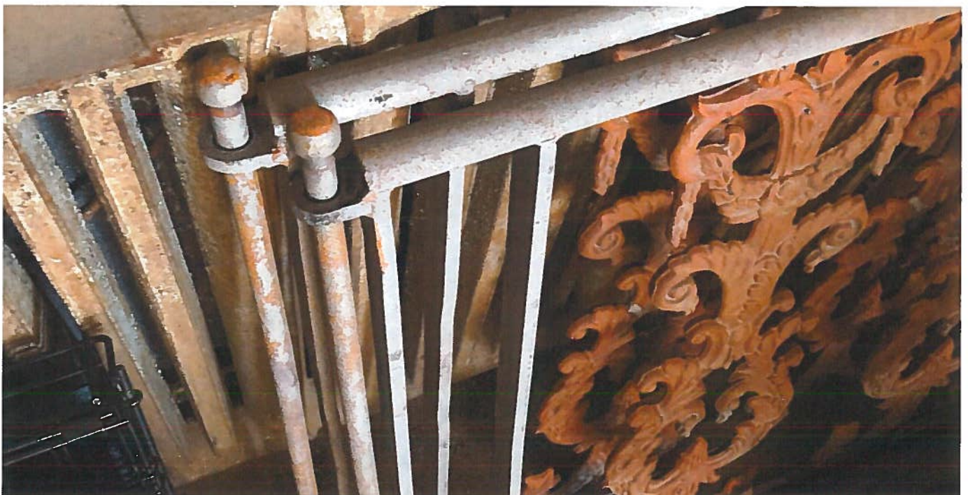
Detailed shot of existing gate.
