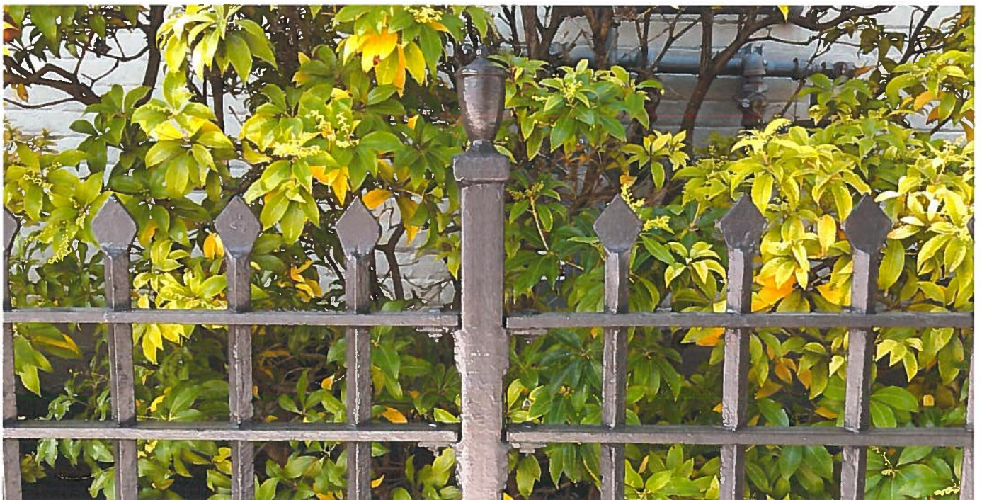
Detailed shot of existing fencing currently installed along the East of the property.
